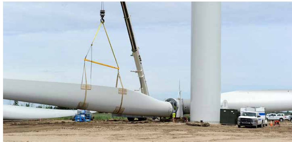
Erecting the wind tower sections, the nacelle, and blades requires dozens of men and multiple cranes working together. Photo provided by DTE Energy.
